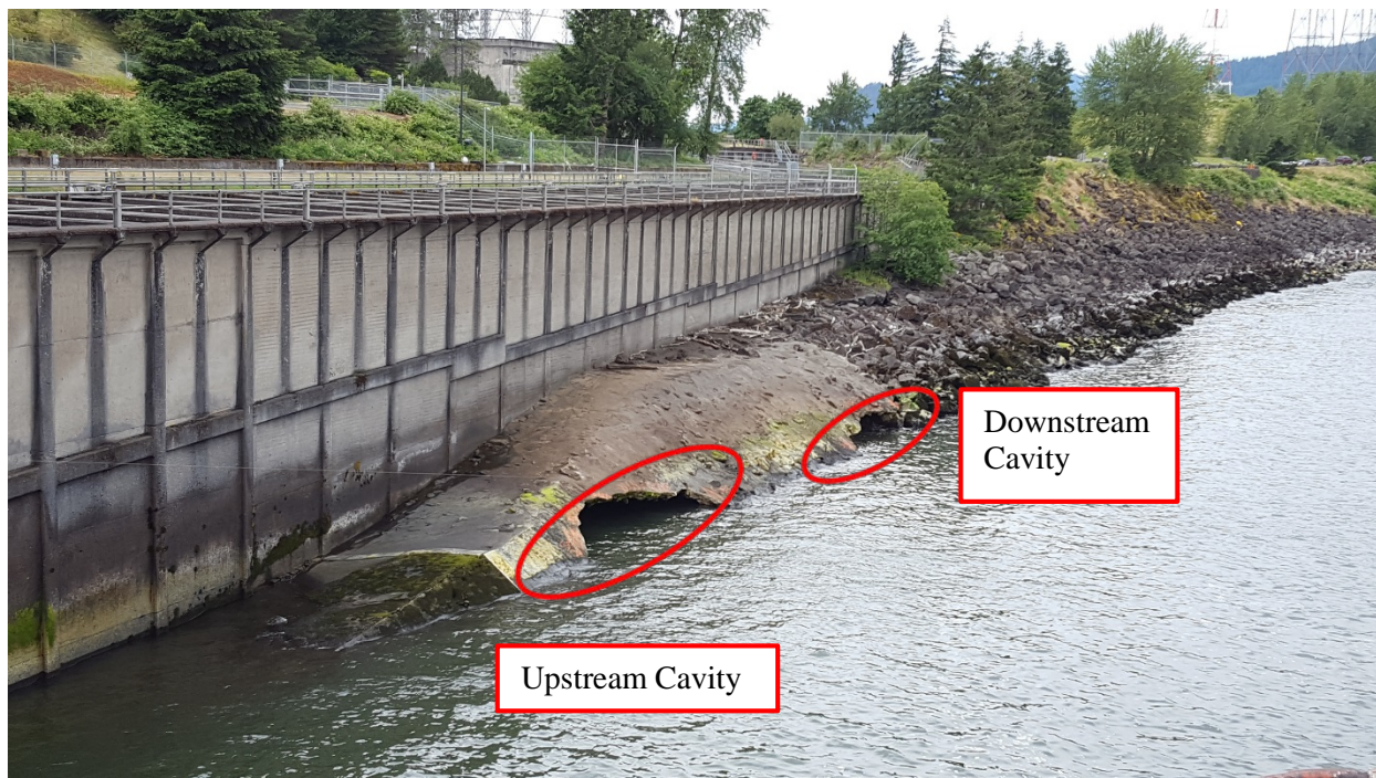
Figure 3-1: Bonneville B-Branch Fish Ladder Erosion Overview Looking West
