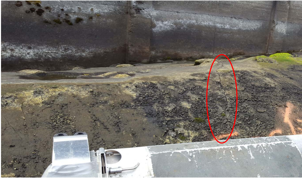
Figure 3-7: Bonneville B-Branch Fish Ladder Grout Apron Stress Fracture
