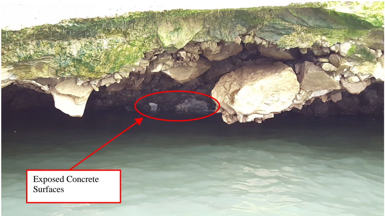
Figure 3-4: Upstream Erosion Looking Inside at Fish Ladder Wall
